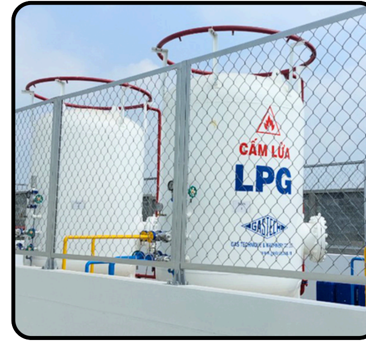
7.5M3 TON TANK - LPG VAPORIZER 200KG/HR
