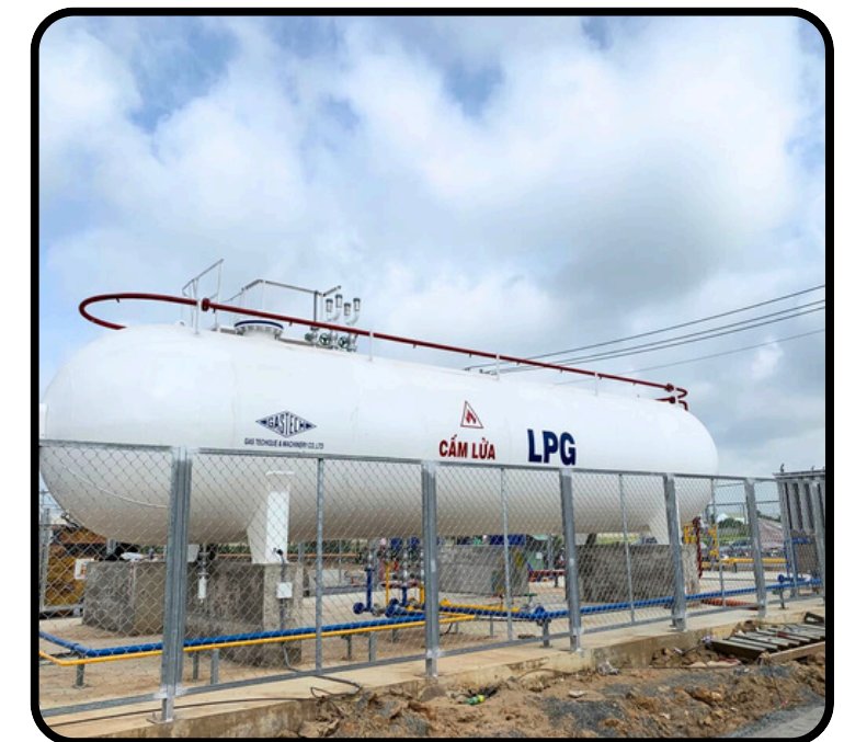
25 TON TANK LPG
