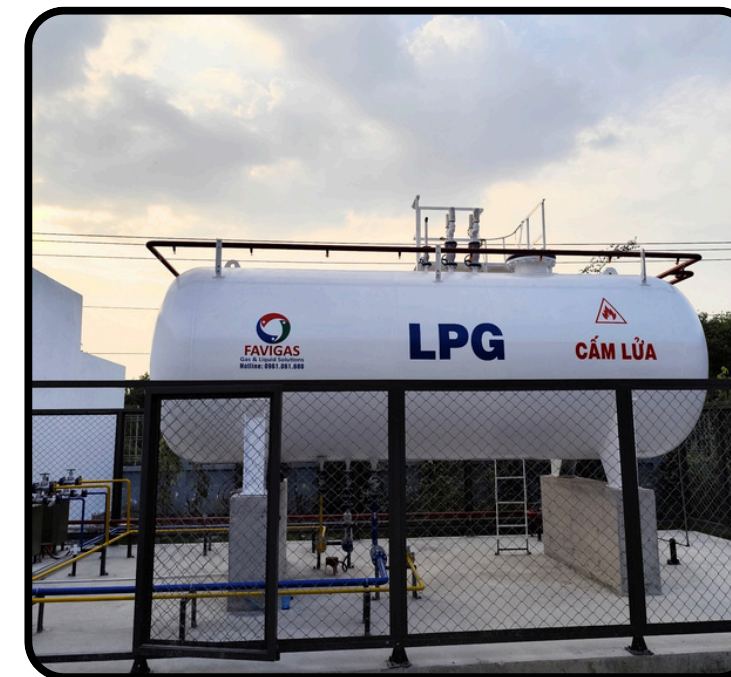
ELECTRIC LPG VAPORIZER AND 10 TON TANK
